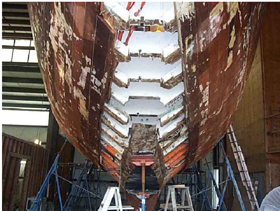
The restoration of Bolero involved removal and replacement of the keel, stem, garboards, and several adjacent planks. Even in this state the beautiful lines of her hull are evident. The hull is double planked with cedar and mahogany over white oak frames.
