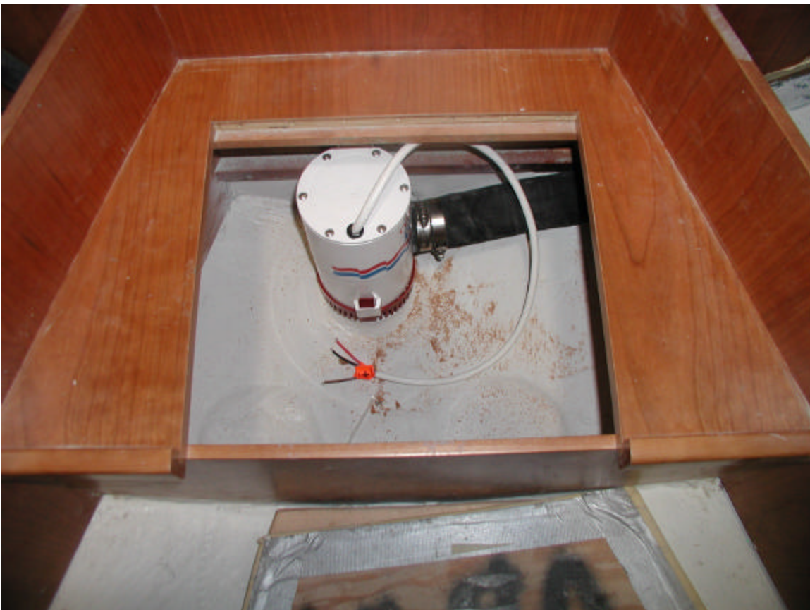
High-capacity bilge pump installed in the forward cabin
