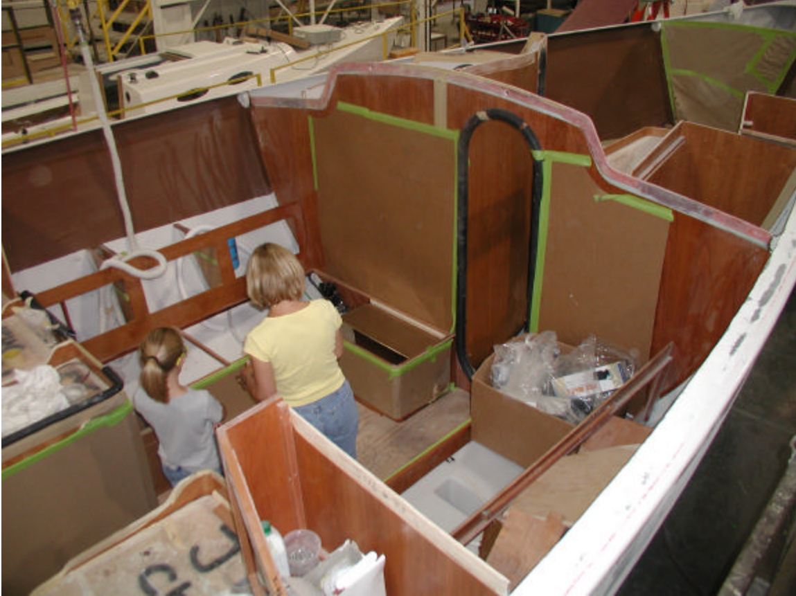
View of the main cabin during construction. The main bulkhead was fitted with a watertight door and silicone seals were installed on all wiring and plumbing passing through this bulkhead.
