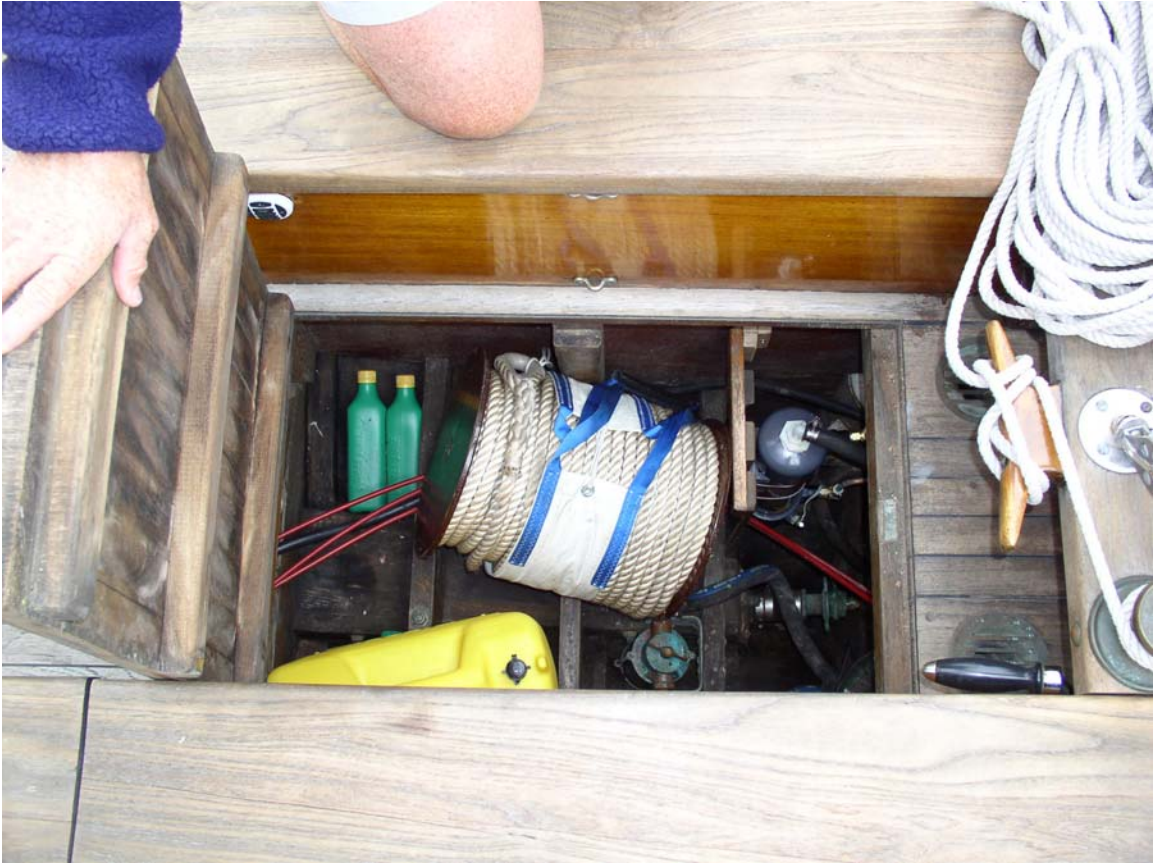
The aft end of the engine can be accessed through a heavy water-tight hatch in the cockpit sole which is gasketed and dogged by a special screw lock. The engine is a 27HP Yanmar. Note the neatly reeled rode for the storm anchor. The fuel capacity is 46 gallons. Three water tanks hold a total of 39 gallons.
