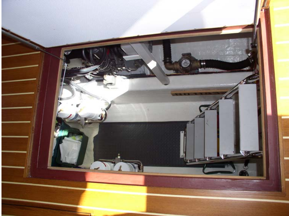
Looking down into the spacious engine room through the counter-balanced hatch at the forward end of the main cabin sole.
