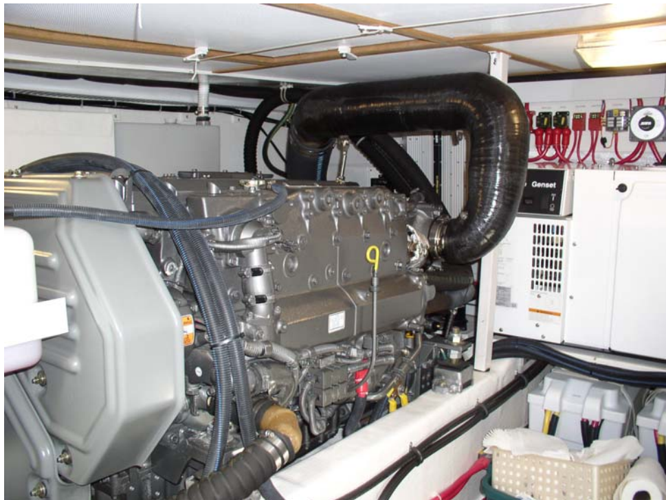
View of the starboard engine looking aft. The Onan genset is mounted on the aft bulkhead.
